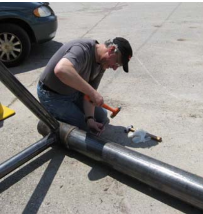
EAA 932 member Steve Mark tapping his name into a leg of the way finding tower after he finished welding on it.
