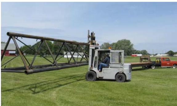
The first completed way finding tower tower being off-loaded during its delivery to the Ultralight Area
